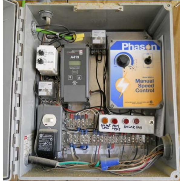
Figure 3: TSC duct system controller
